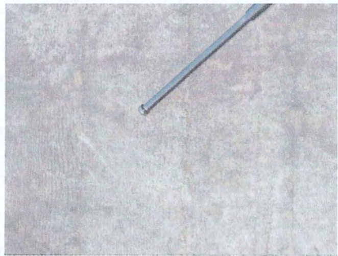
Scratch marks below suspected exit point.. Approximately 6' off bottom
